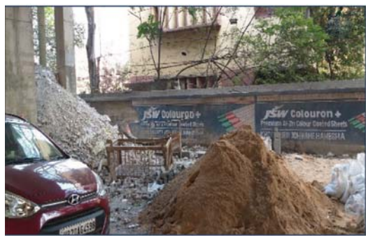
Plate 6: Dumping of construction material at footpath and blocking of footpath near Thakurpukur
